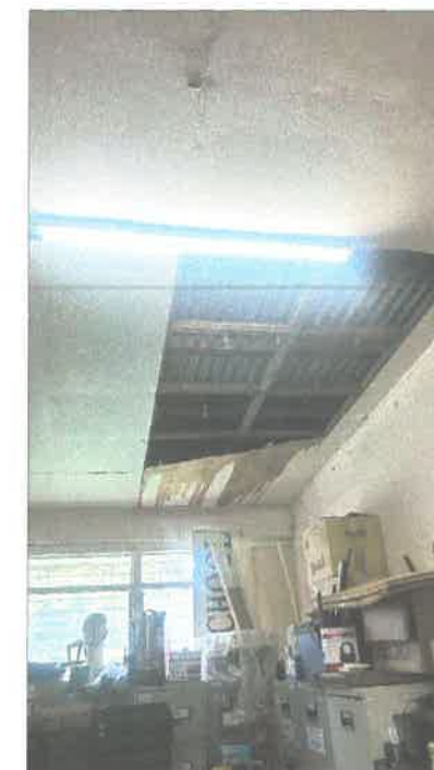
Existing UBA Office storage room with dilapidated ceiling( above)
